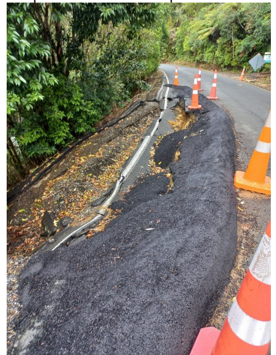
Right: Example of bunding on road surface on Kellys Road, which will channel rain water on the road past the slip.
